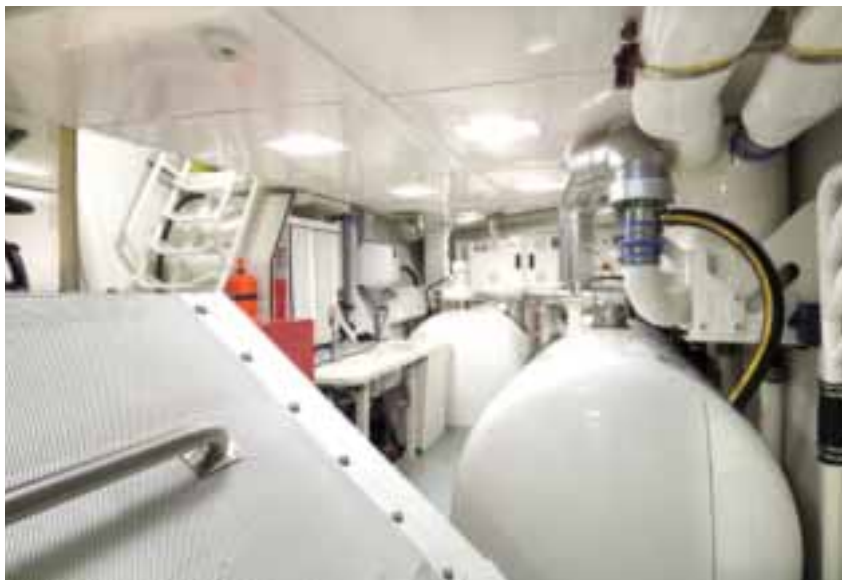
LEFT: THE ANGLED WATERTIGHT BOX, FAR LEFT, CONTAINS ONE OF THE RETRACTABLE SWINGING THRUSTERS.
